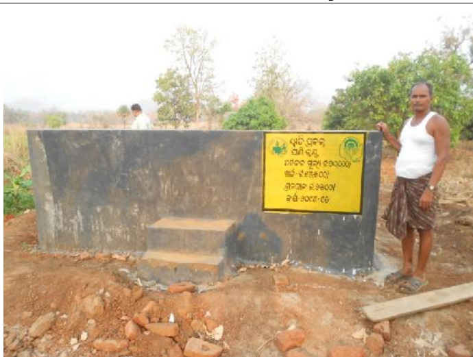
Water storage Tank at WADI field for irrigation
